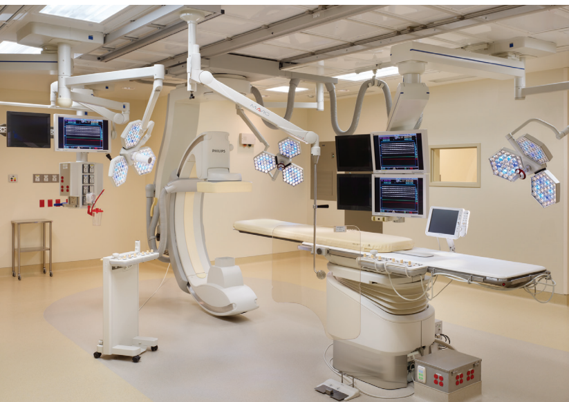
Figure 2: Hybrid Operating Room
